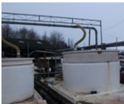
Anaerobic digester at Bank Farm
